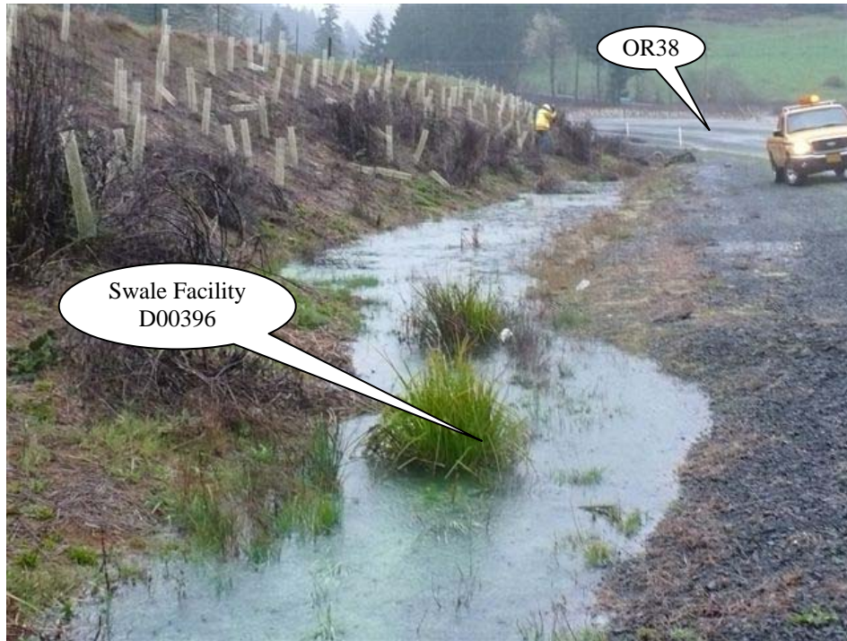
Photo 3: Looking east, storm flow generated from OR38 on the right side of the picture contributes stormwater into the swale. Stormwater is flowing from the bottom of the picture towards the top of the picture.
