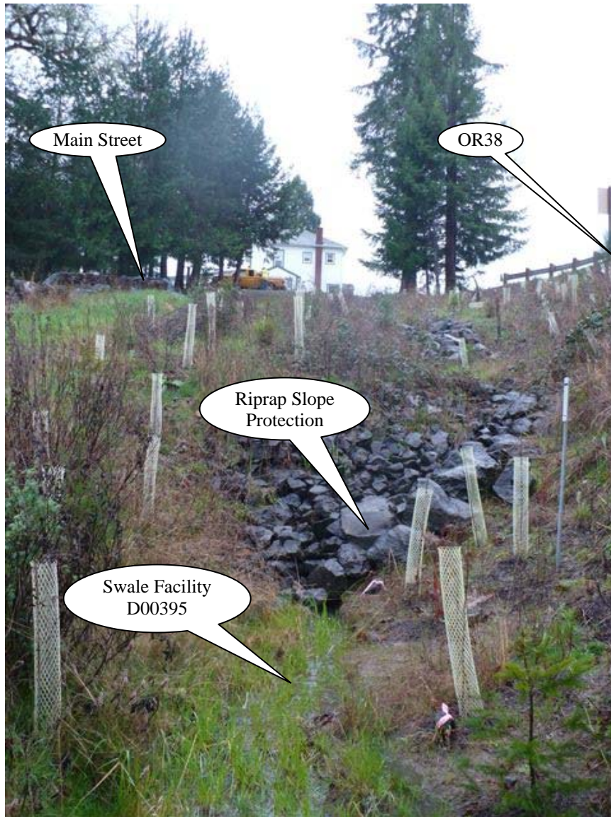
Photo 3: Looking west, storm flow from the Elk Creek Bridge discharges on the riprap slope shown in the upper portion of the picture. The stormwater enters the swale at the base of the riprap slope and flows towards the bottom of the picture.
