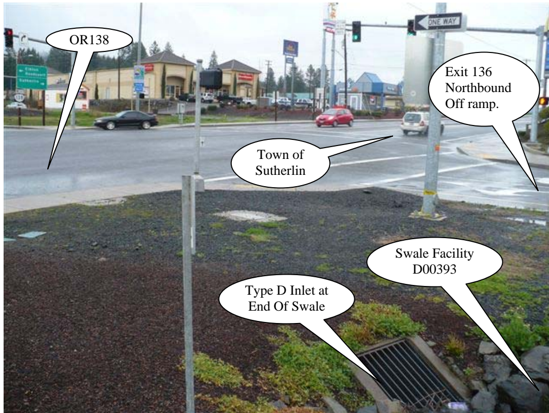
Photo 2: Looking north, flow from the swale is collected in the Type -D inlet/outlet control structure shown.
