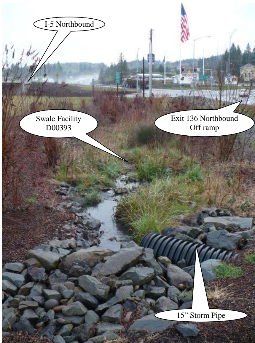
Photo 3: Looking north. The 15-inch culvert, located at the bottom of the picture, contributes flow at the facility inlet. Sheet flow from I-5 Northbound travel lanes and the Exit 136 northbound off ramp also contribute flow. Water is flowing towards the top of the picture.
