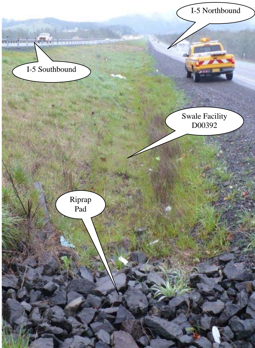
Photo 2: Looking north, flow into the swale is generated from the sheet flow originating on the northbound and southbound travel lanes of I-5. Water is collected at the riprap pad and flows towards the top of the picture.
