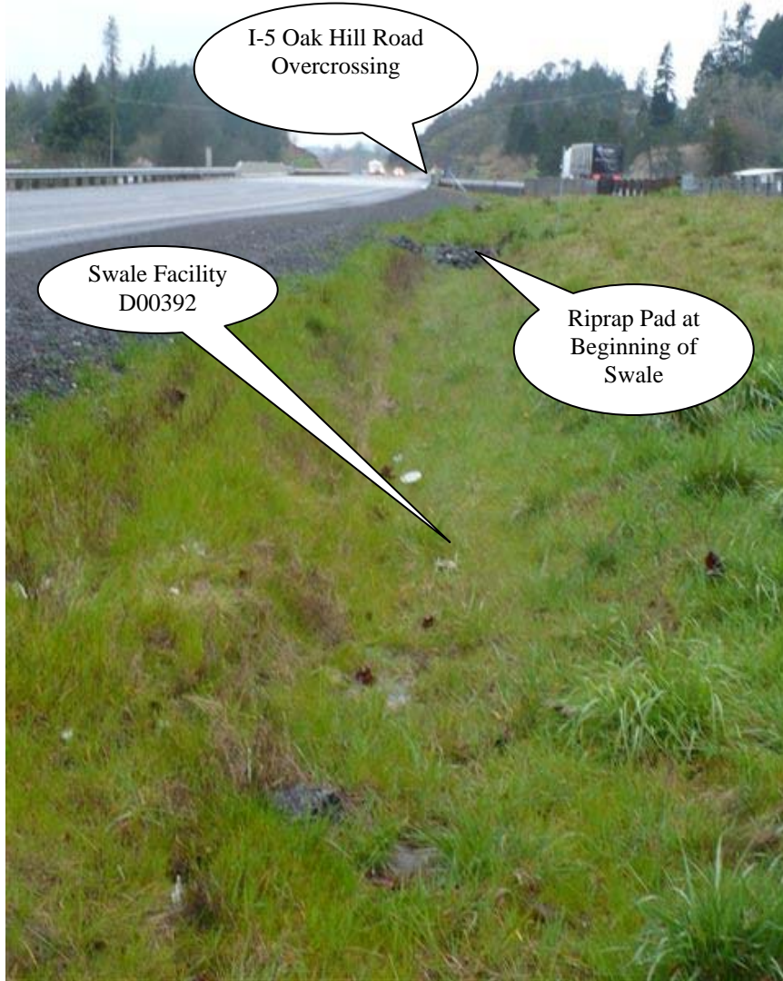
Photo 1: Looking south, flow into the swale is generated from the sheet flow originating on the northbound and southbound travel lanes of I-5. Water is flowing towards the bottom of the picture.
