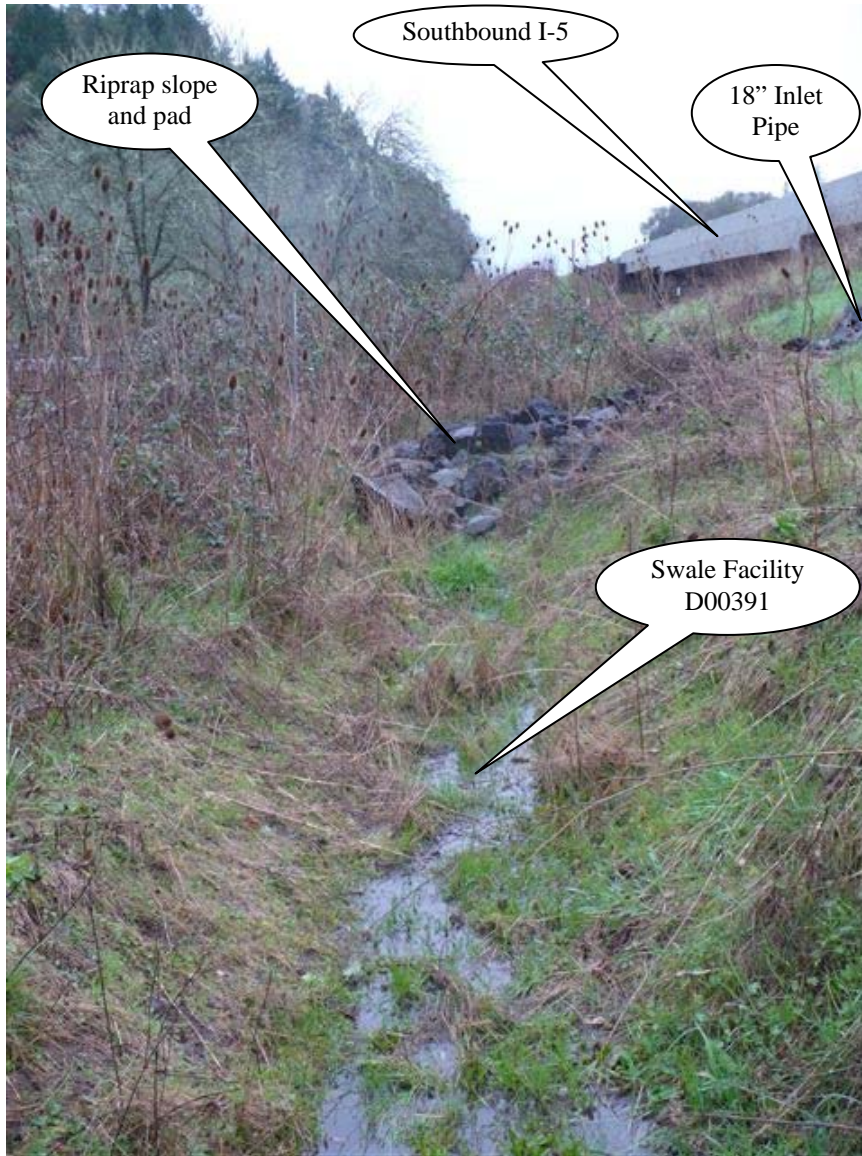
Photo 2: Looking north, flow into the swale is generated from the 12-inch inlet pipe. Water is collected at the riprap pad and flows towards the bottom of the picture.
