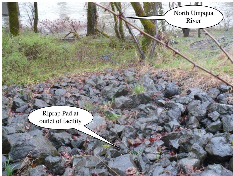
Photo 3: Looking north, the riprap pad shown is located at the outlet of the swale as an erosion control measure.
