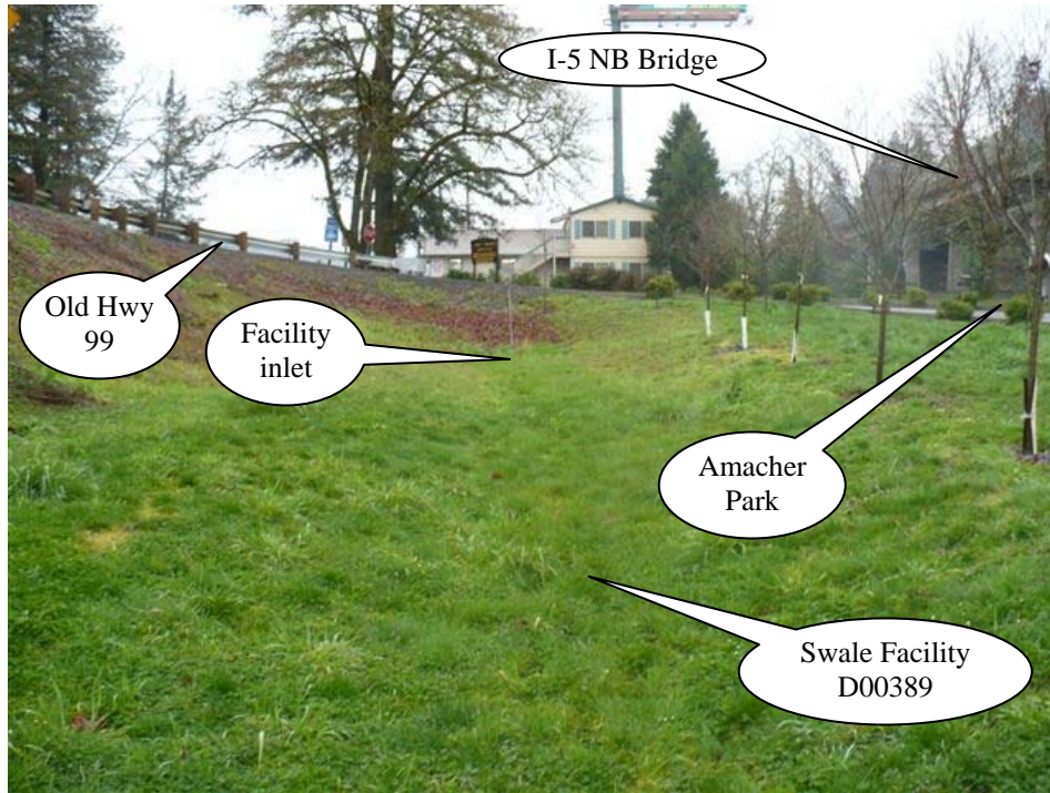
Photo 2: Looking south, the Type G-2 facility inlet is shown towards the upper portion of the picture. Water flows towards the bottom of the picture.
