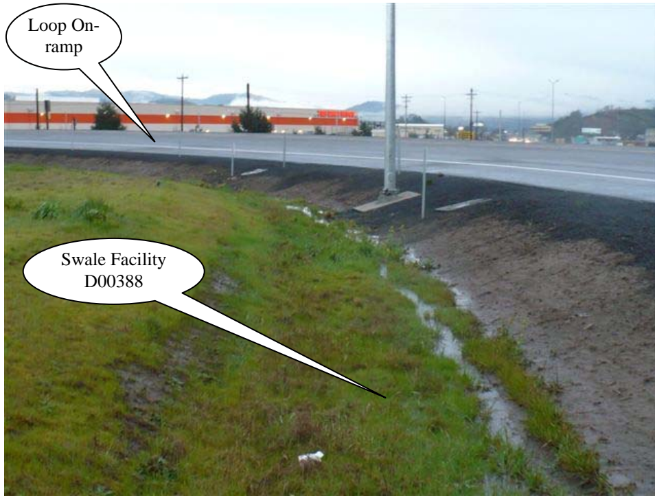
Photo 1: Looking east, flow into the swale is generated from the northbound loop on-ramp shown in the picture. Water is flowing towards the bottom of the picture.
