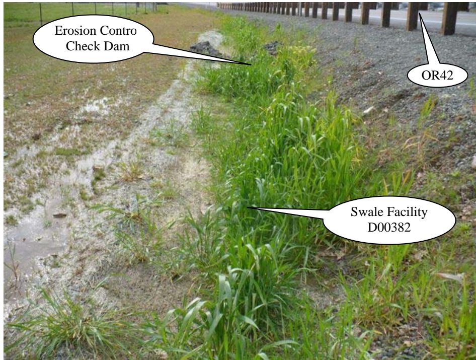
Photo 2: Looking west, sheet flow from OR42 on the right side of the picture contributes stormwater into the swale.
