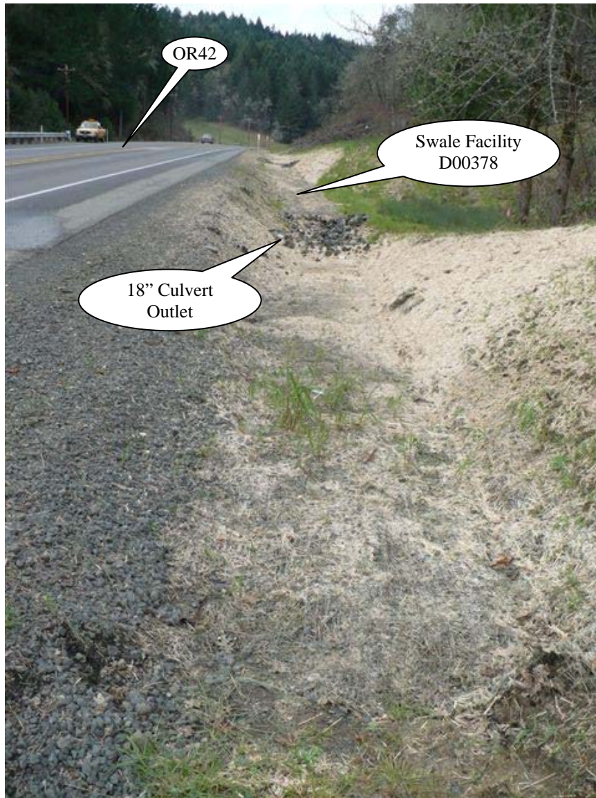
Photo 1: Looking west, sheet flow from OR42 on the left side of the picture contributes stormwater to the swale.
