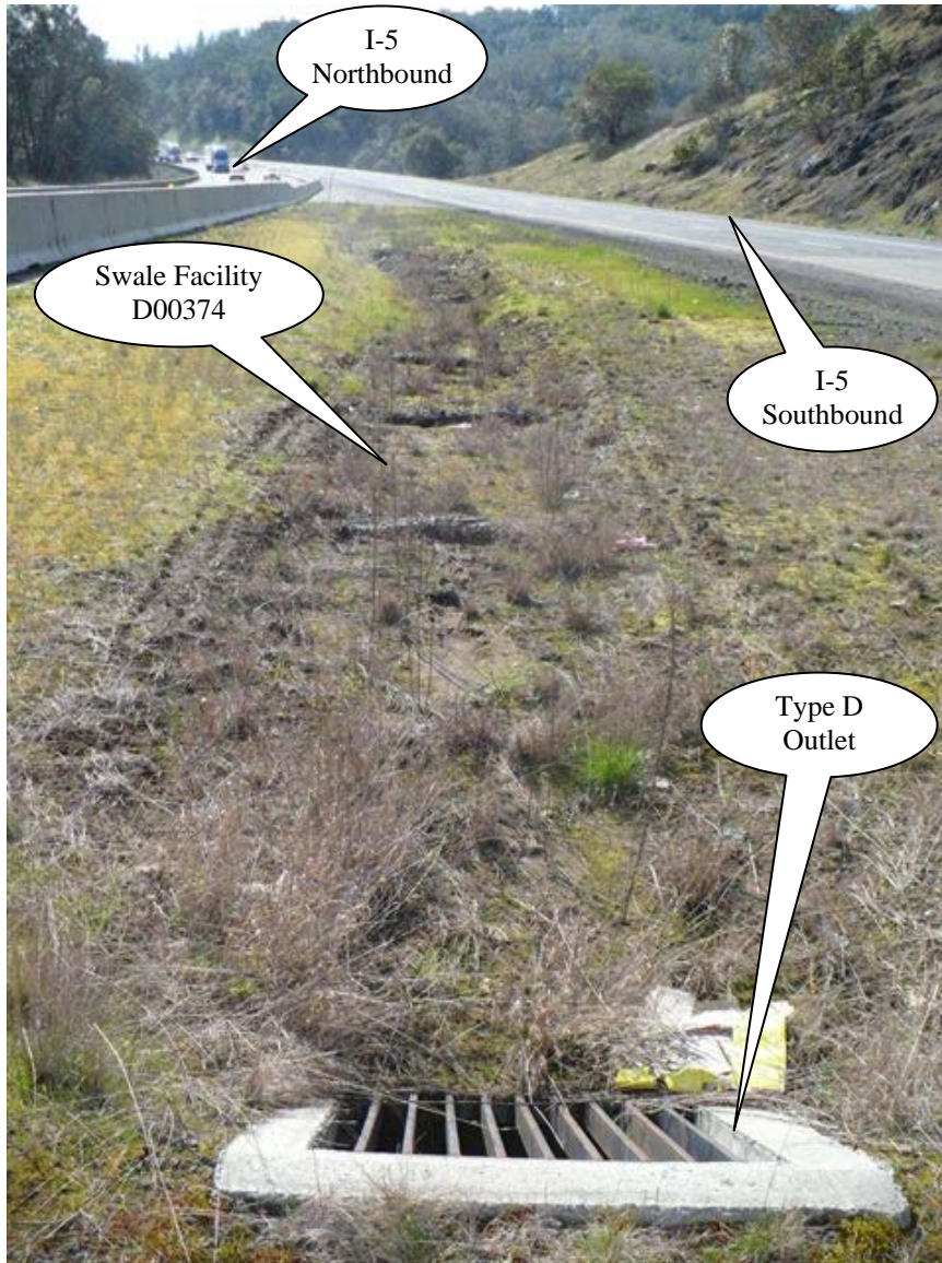
Photo 1: Looking south, flows enter the swale when generated from the north and southbound lanes of I-5. The Type-D inlet/outlet functions as the facility outlet.
