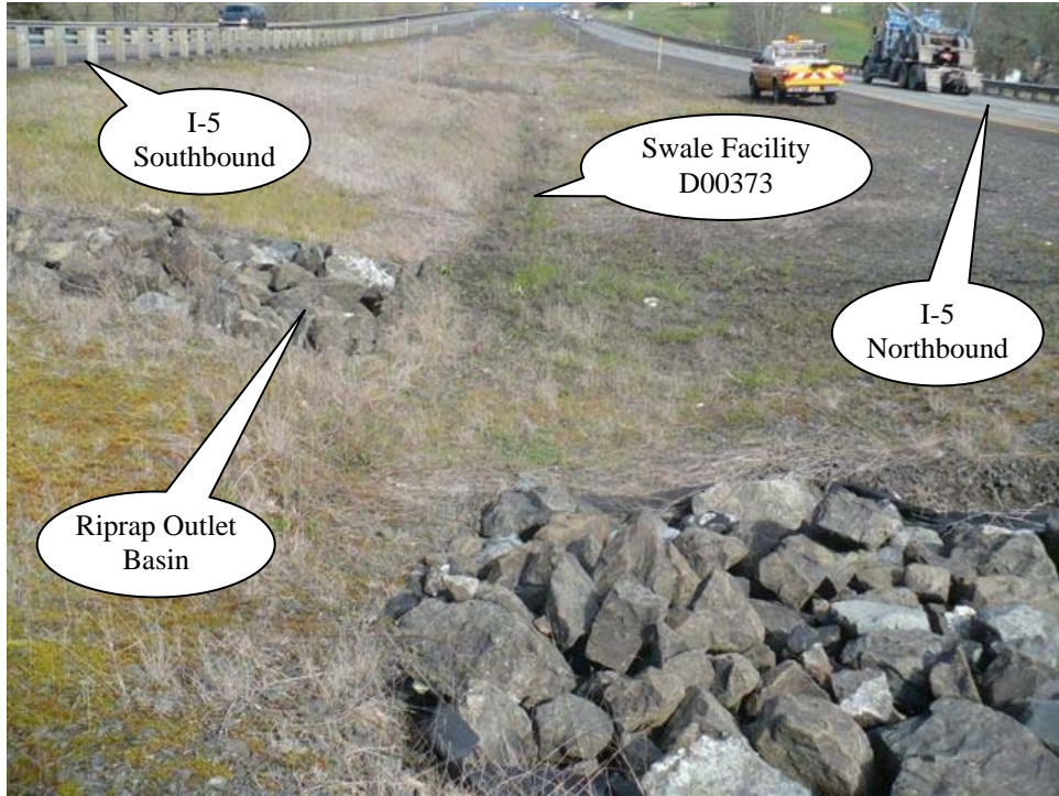
Photo 1: Looking north, flow into the swale is generated from I-5 shown on the left and right side of the picture. Riprap basins shown at the bottom of the picture function to infiltrate flow and dissipate energy.
