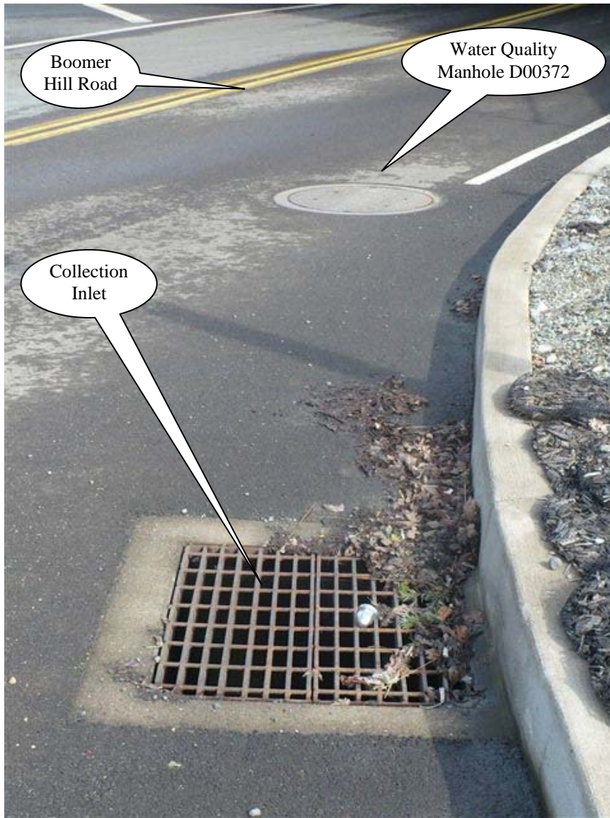
Photo 3: Photo looking south with the collection inlet shown at the bottom of picture. Flow is conveyed directly from this inlet to the water quality manhole shown in the upper portion of the picture.
