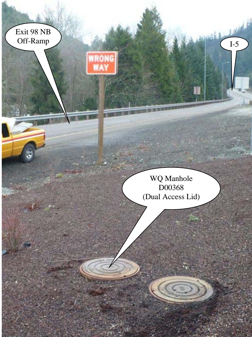
Photo 1: Looking south. The dual access manhole lids for the water quality manhole are shown, in the foreground.
