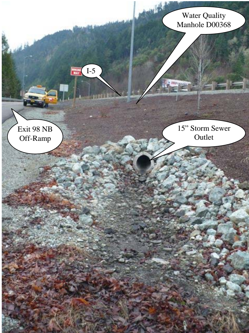
Photo 4: Looking south, at the outlet ditch with the 15-inch storm sewer outlet shown in the foreground. The treated water flows to this ditch from the water quality manhole shown in the upper portion of the picture.
