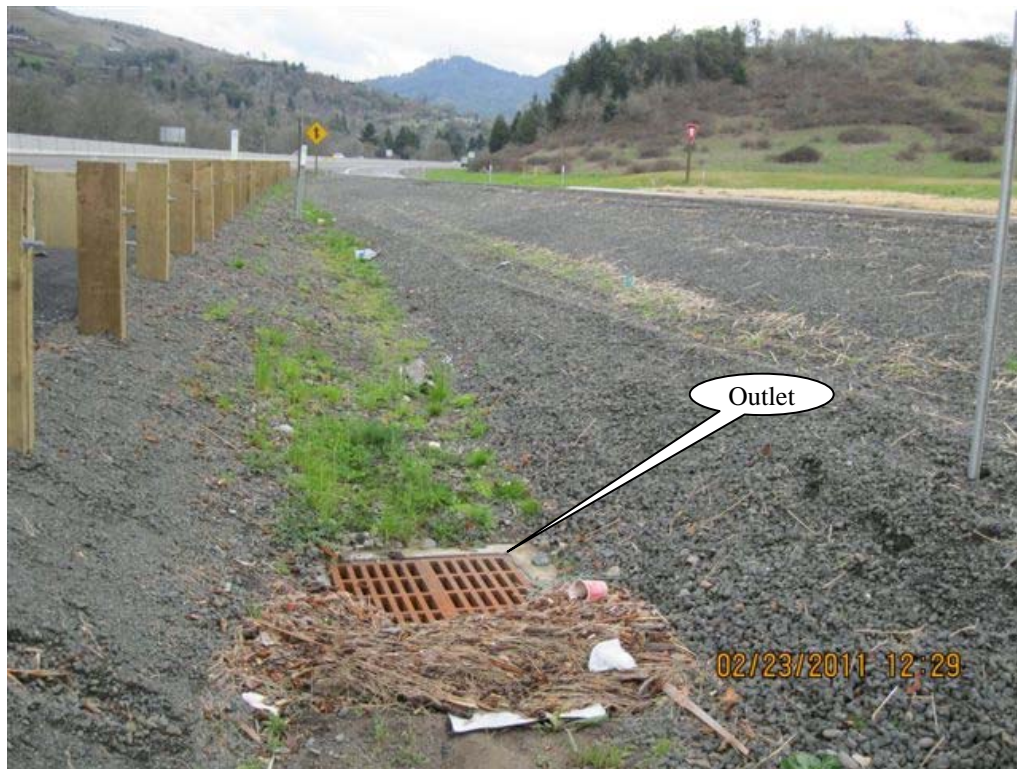
Photo 2: Type G2-MA swale outlet located in the gore between the weigh scale on-ramp and the southbound lanes of I-5.
