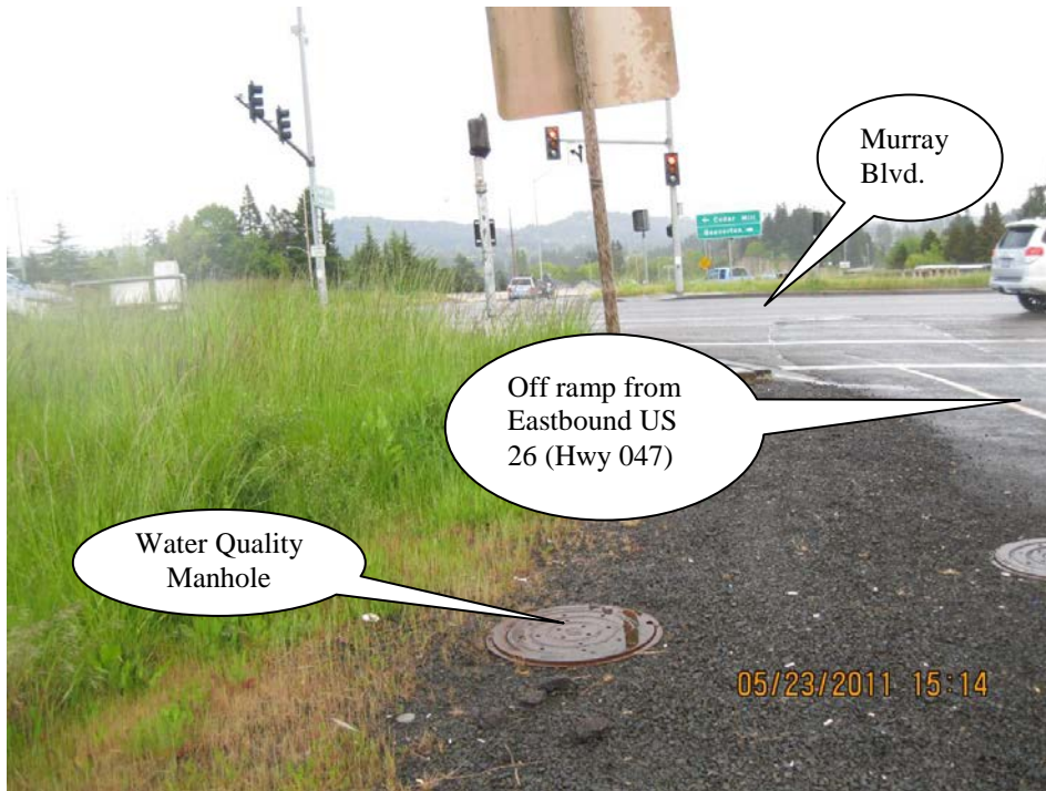
Photo 1: Water Quality Manhole, looking eastbound toward Murray Blvd and the ramps, leading to and from US 26 (Hwy 047).
