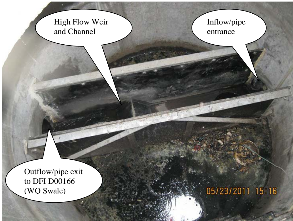
Photo 2: Water Quality Manhole, showing the entrance and exit pipes, the high flow weir and channel, and the treatment sump, below.
