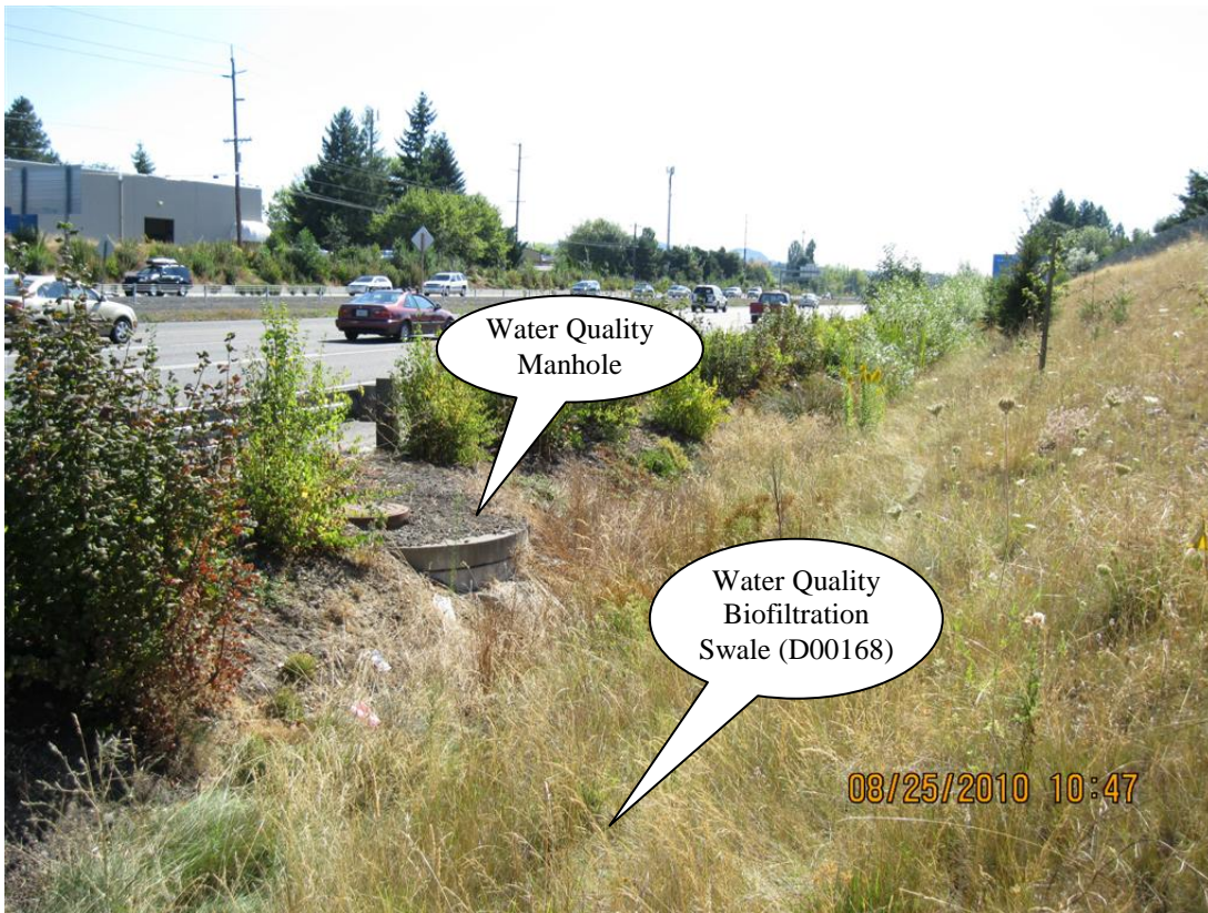
Photo 1: Water Quality Manhole looking east on US 26.
