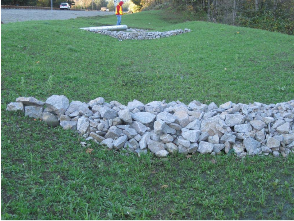
Photo 1: Looking west at the facility inlet and a flow spreader. The highway (I-84) is on the left.
