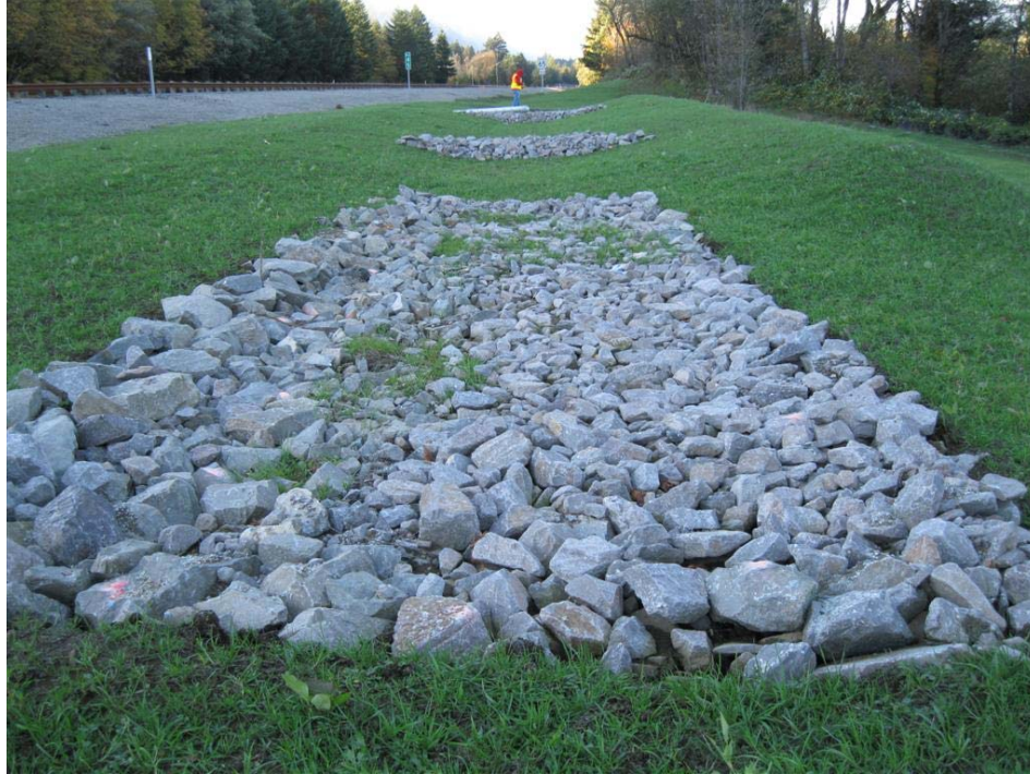
Photo 3: Looking west toward the facility inlet from the riprap pad near the outlet.
