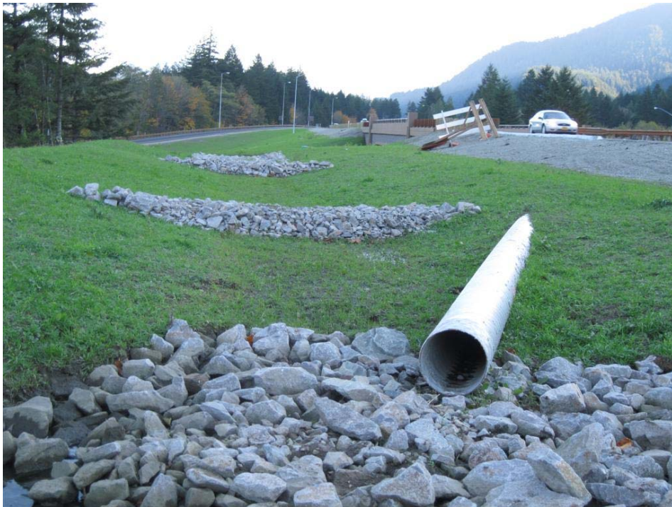
Photo 2: Looking east from the facility inlet toward the flow spreaders and facility outlet.
