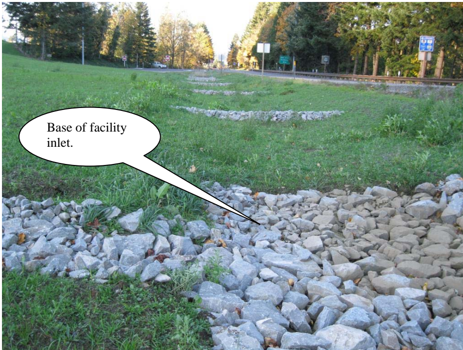
Photo 2: Water quality facility inlet and flow spreaders, looking west. Off-ramp located to the right.
