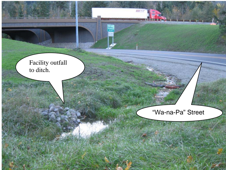
Photo 5: Water quality facility outfall to ditch looking south toward I-84.
