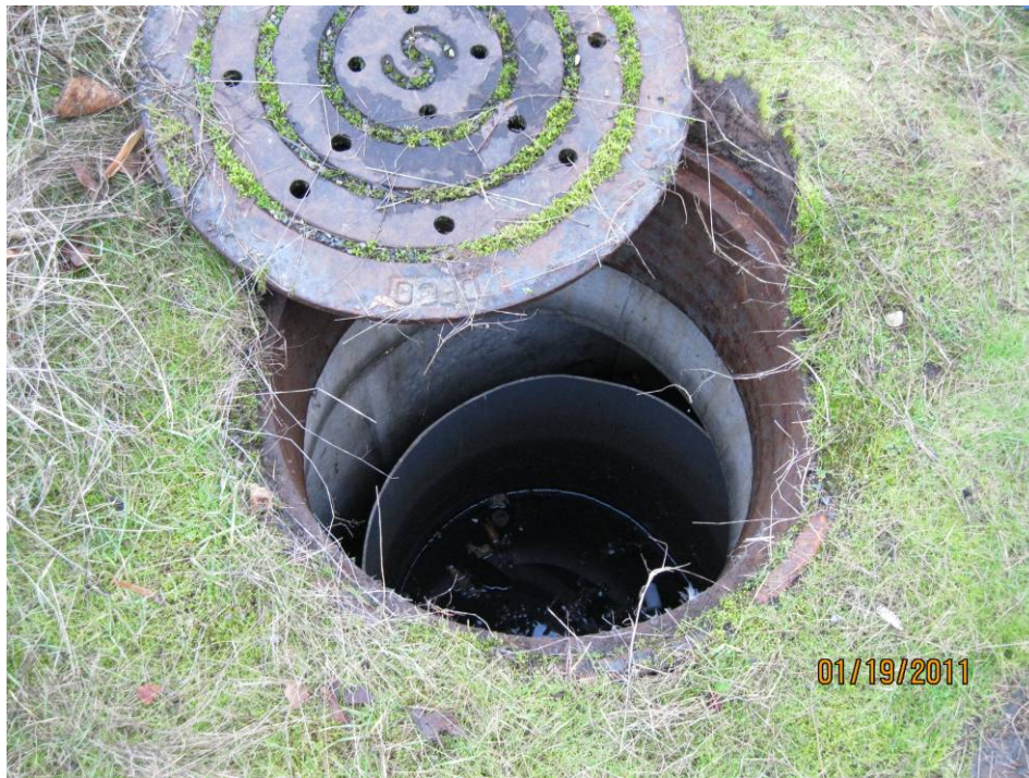
Photo 2: Looking into the water quality manhole through one of its access lids. It appears this manhole may need retrofitting to allow for greater clearances, facilitating easier maintenance.
