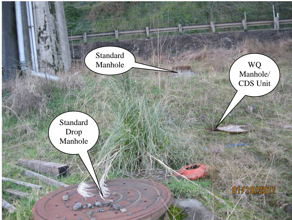
Photo 2: Looking southwest from beneath St. Johns Bridge toward the water quality manhole facility and St. Helens Road.
