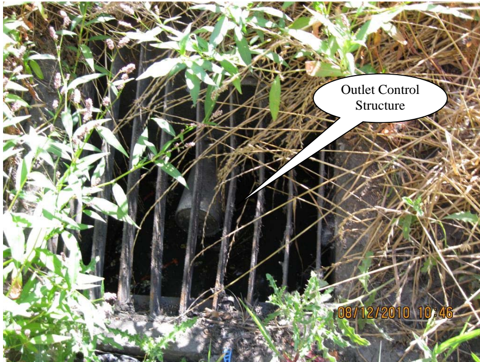
Photo 5: Close up of water quality outlet of the outlet control structure. Outlet piping is visible.
