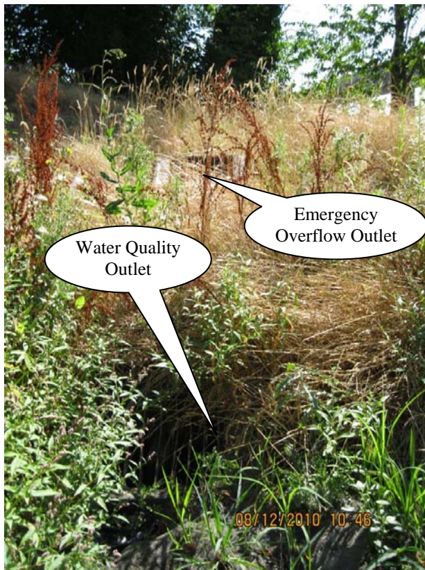
Photo 6: Outlet control structure, including both the water quality outlet and the emergency overflow outlet.
