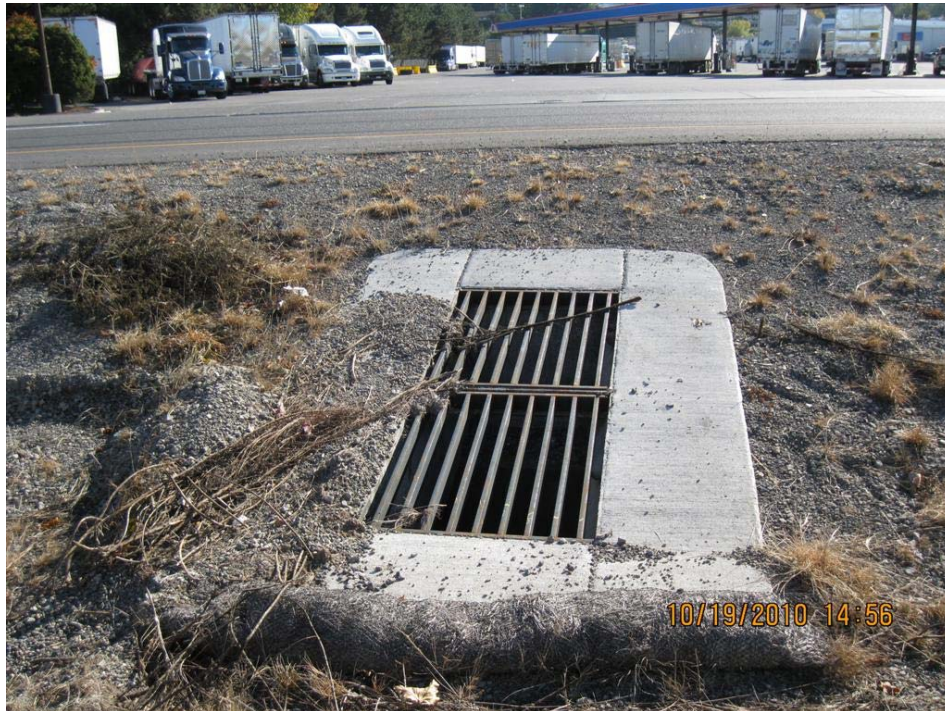
Photo 5: Looking south at outlet structure from the facility's furthest-most point west. This Type M-E inlet/outlet at Point C replaced an existing inlet and ties to an existing system, flowing eastward.
