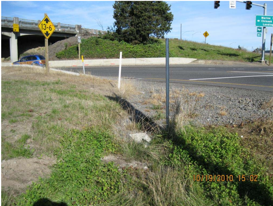
Photo 3: Culvert paved-end slope facility inlet at Point D, looking northeast while at the intersection of NW Frontage and Graham Roads.
