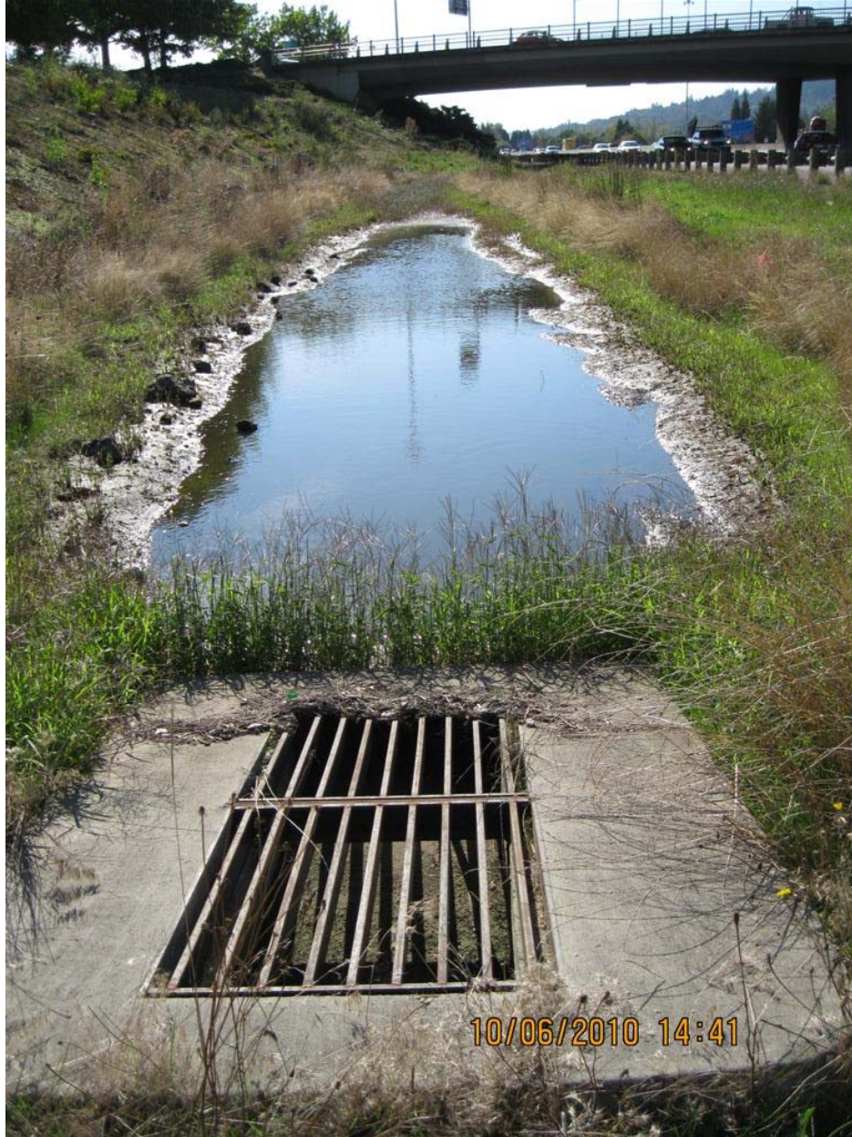
Photo 1: Looking west at the water quality swale and its outlet structure, Point C.
