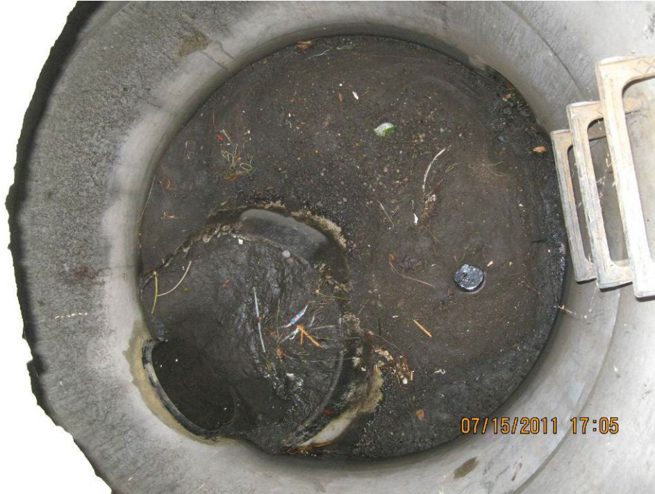
Photo 2: Interior view of Stormceptor water quality manhole, completely silted over and needing maintenance to function properly.
