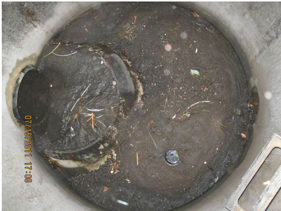
Photo 3: Interior view of Stormceptor water quality manhole, completely silted over and needing maintenance to function properly.
