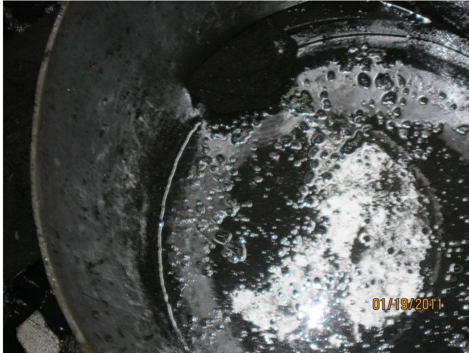
Photo 3: Internal view of water quality manhole, showing some need of .maintenance.
