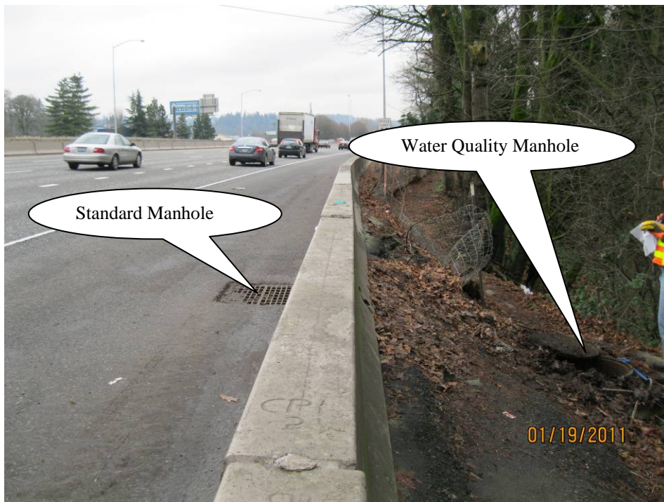
Photo 2: Looking south at both the standard manhole and the water quality manhole.
