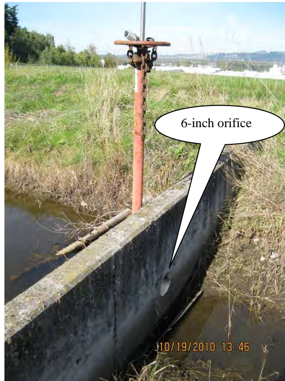
Photo 6: Looking northwest at sluice gate and headwall 2 at the end of Pond No. 1; Point D of Operational Plan, Appendix A.
