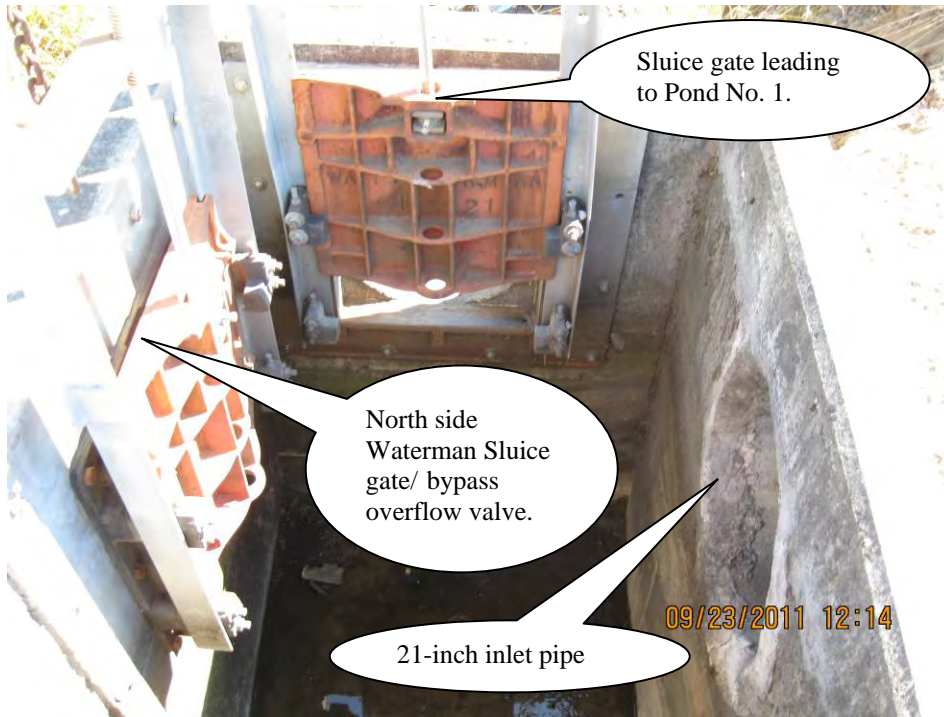
Photo 4: Internal view of diversion box (sediment vault), sluice gate and headwall at the facility inlet; Points A and B of Operational Plan, Appendix A.
