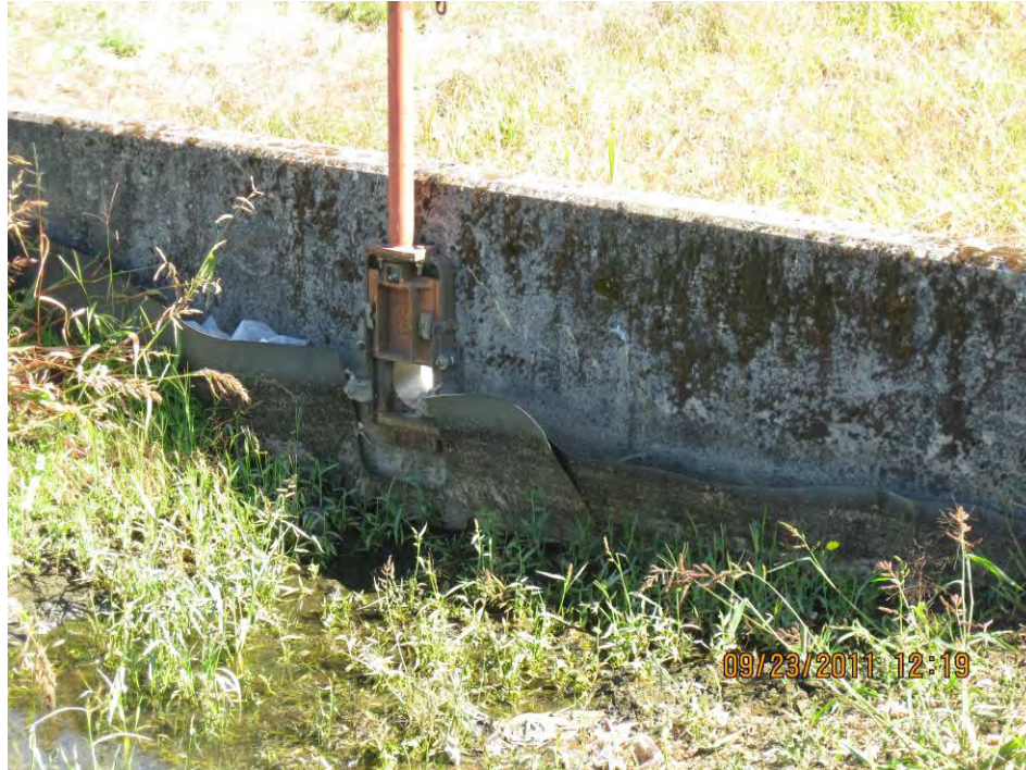
Photo 7: Looking northwest at sluice gate and headwall 2 at the end of Pond No. 1; Point D of Operational Plan, Appendix A. This is a more recent view than earlier photos, showing how the pond's bottom is lower than was originally designed.
