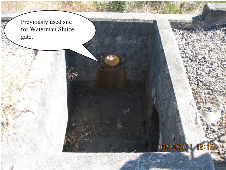
Photo 9: Looking eastward into the diversion box (sediment vault) near the facility outlet; Points H & I.
