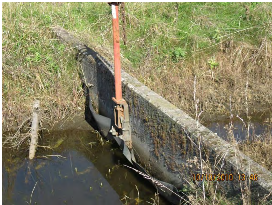
Photo 5: Looking northeast at sluice gate and headwall 2 at the end of Pond No. 1; Point D of Operational Plan, Appendix A.
