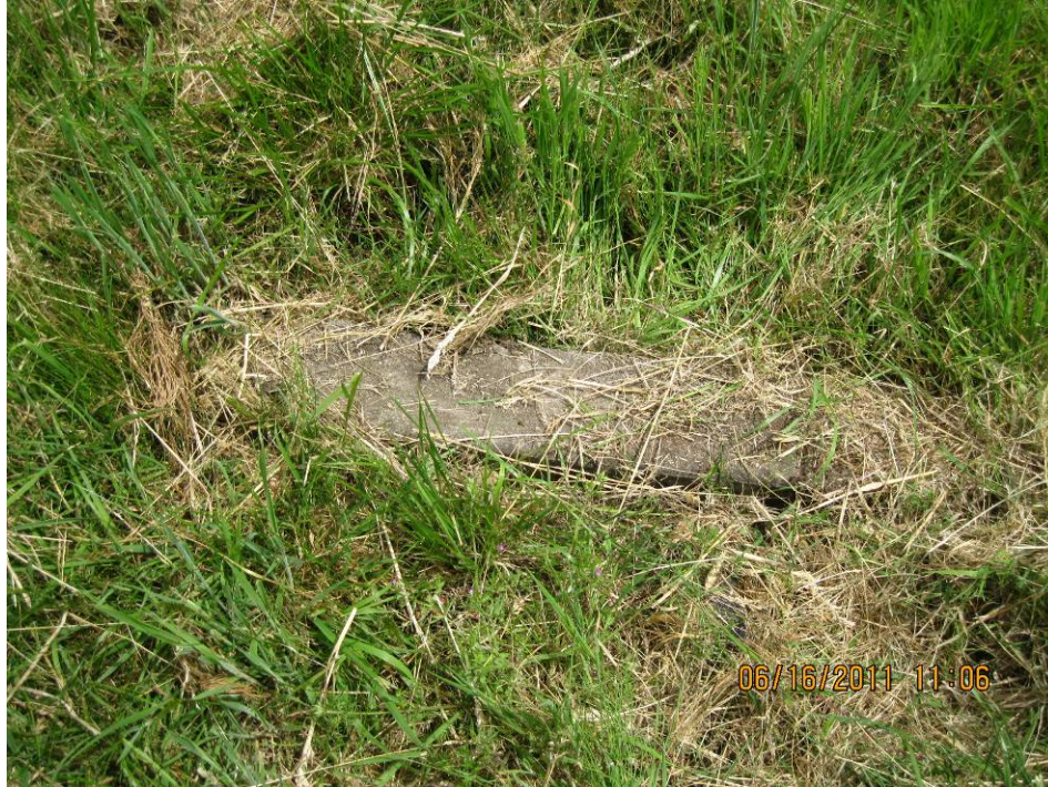
Photo 3: Looking at the concrete knee wall near the entrance to the swale. Hwy 92 is located to the right.
