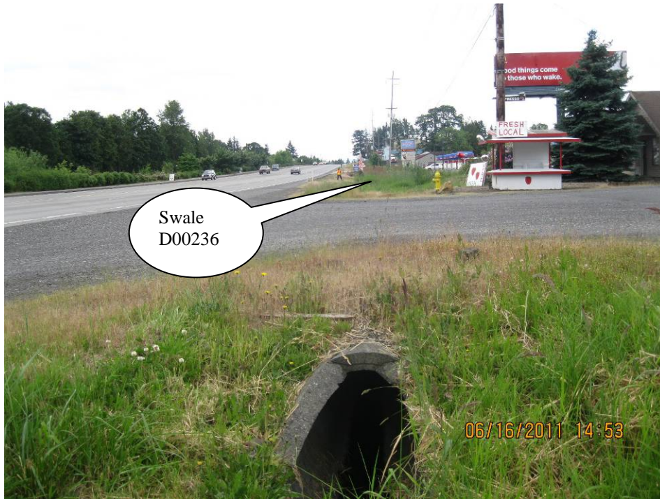
Photo 1: Looking south toward a culvert entrance to the swale with the swale being located on the opposite side of the driveway shown.
