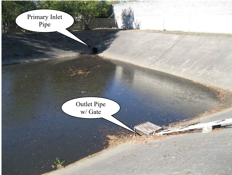
Photo 2: Detention pond primary inlet and outlet.
