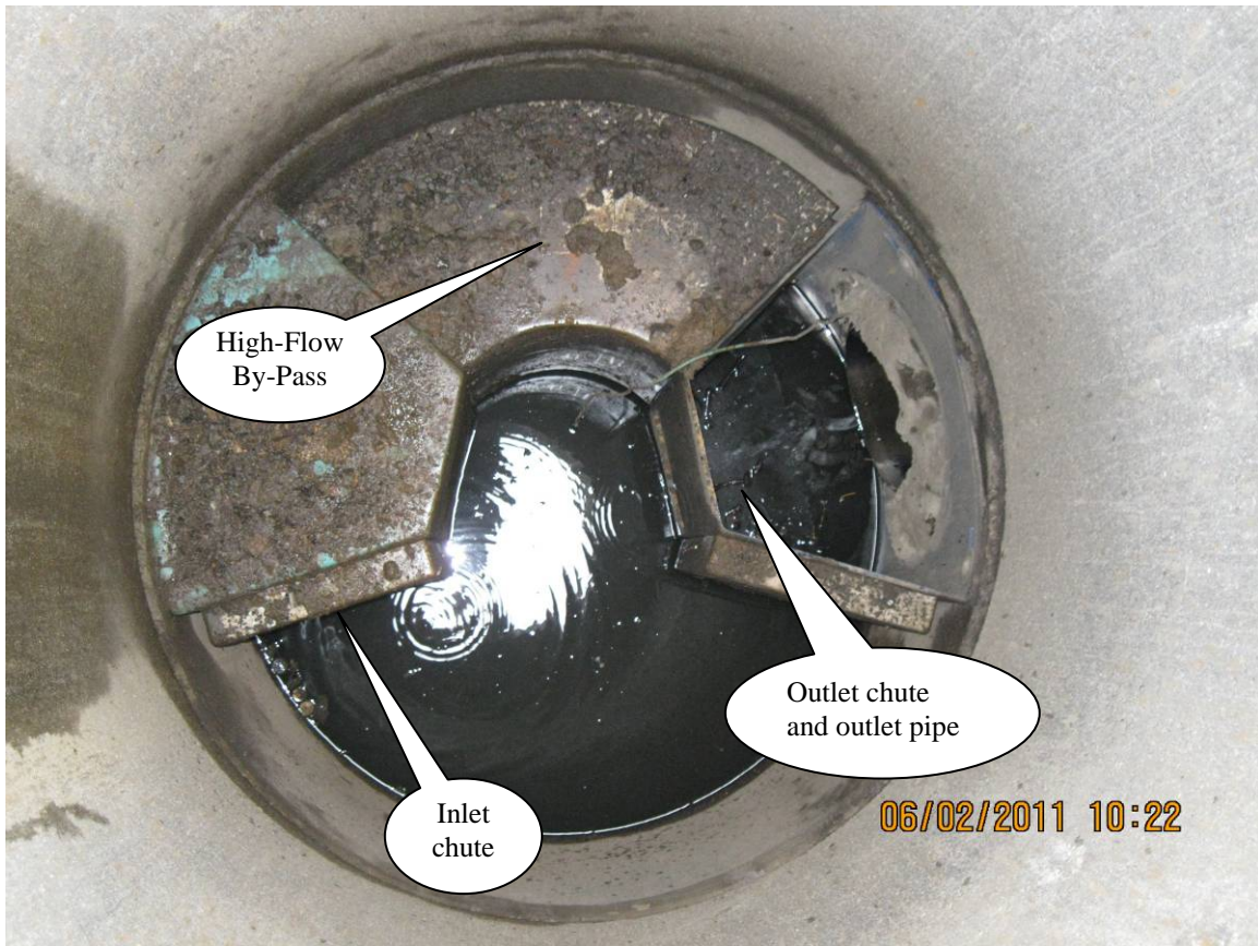
Photo 1: Interior view of water quality manhole.
