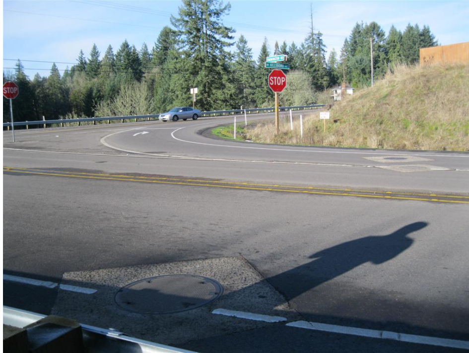
Photo 2: Looking northwest at water quality and flow control manhole structures.
