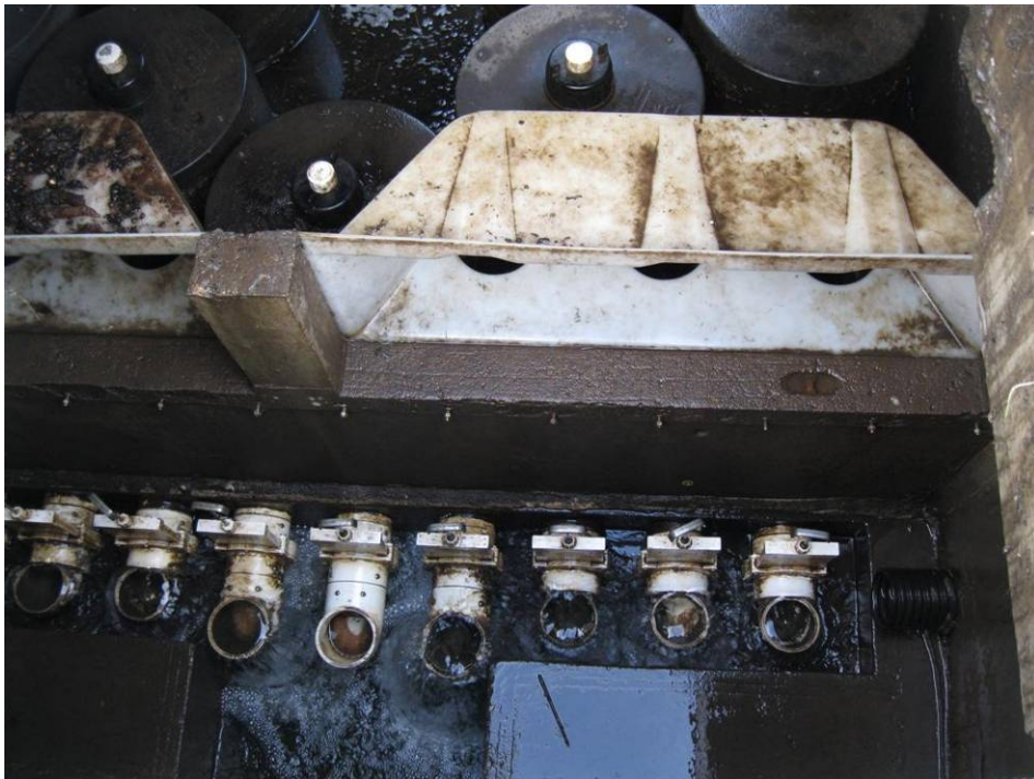
Photo 3: Zoomed in view of the outlet to the retrofitted StormFilter System, showing the under drain pipes, remaining in use from the previous design installation.
