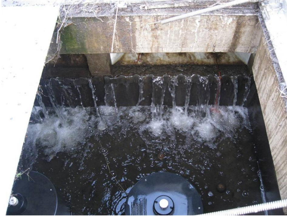
Photo 2: Zoomed in view of the inlet to the StormFilter System. The Compost Stormwater Filter has been retrofitted with StormFilter cartridges from Contech Products, Inc.
