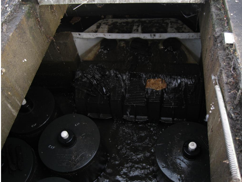
Photo 2: Zoomed in view of the inlet to the StormFilter System. The Compost Stormwater Filter has been retrofitted with StormFilter cartridges from Contech Products, Inc.
