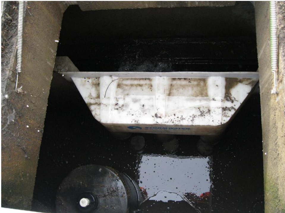
Photo 3: Zoomed in view of the outlet to the StormFilter System.
