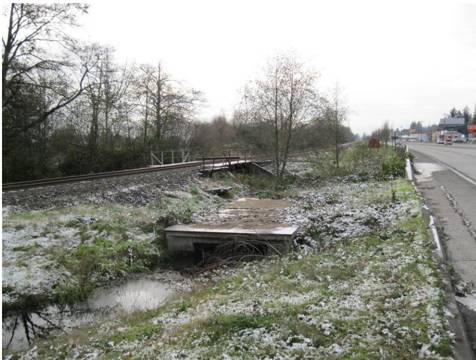
Photo 1: Looking south at the facility inlet and opening to the vault's inlet bay.
