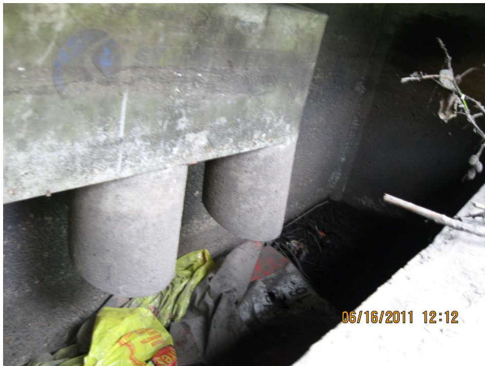
Photo 5: View of the riser pipes/inlet hood with debris seen in inlet bay.
