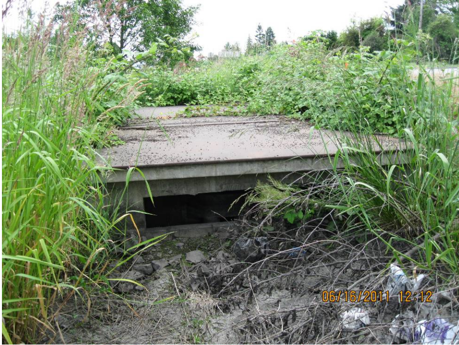
Photo 2: View of the facility inlet and vault opening, riser pipes and inlet bay.
