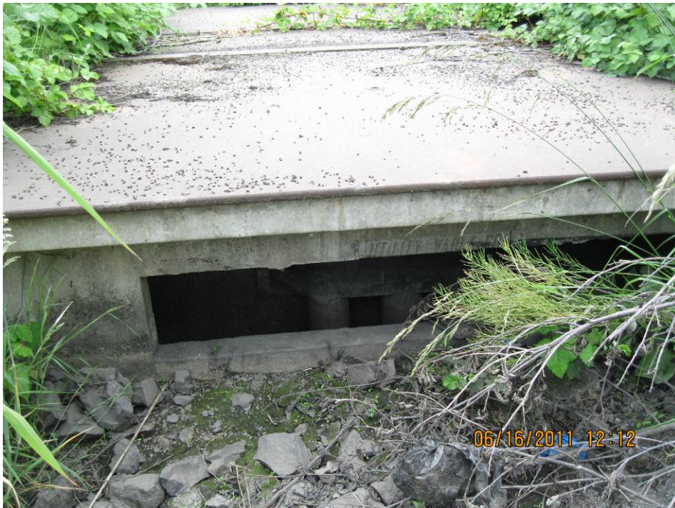
Photo 3: Closer view of the facility inlet, vault's riser pipes/inlet hood and inlet bay.
