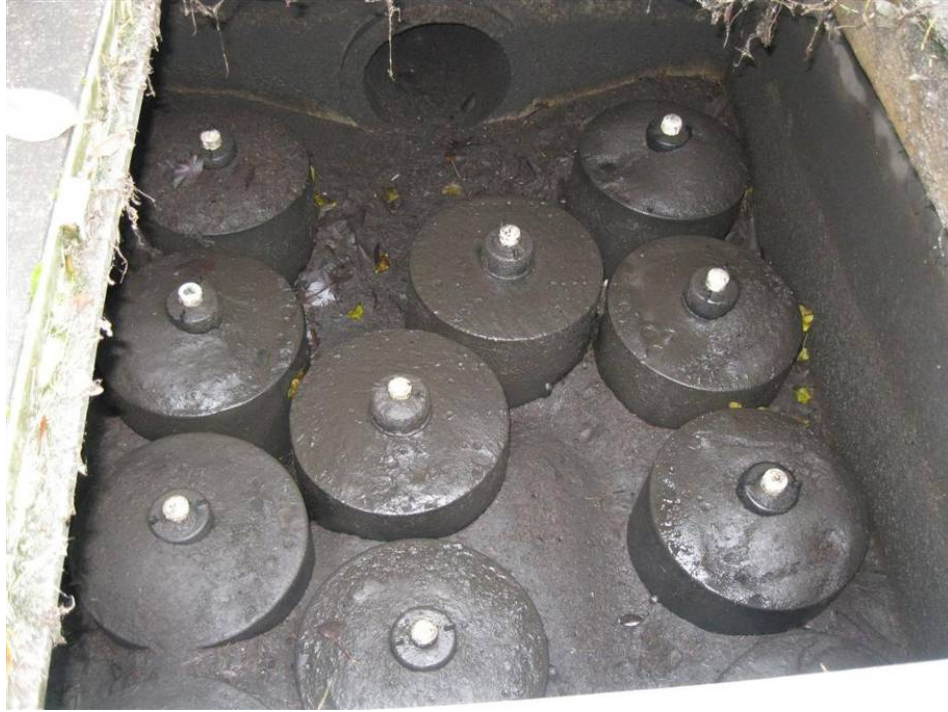
Photo 2: Looking inward at the radial filter cartridges – entrance to Vault 2.
