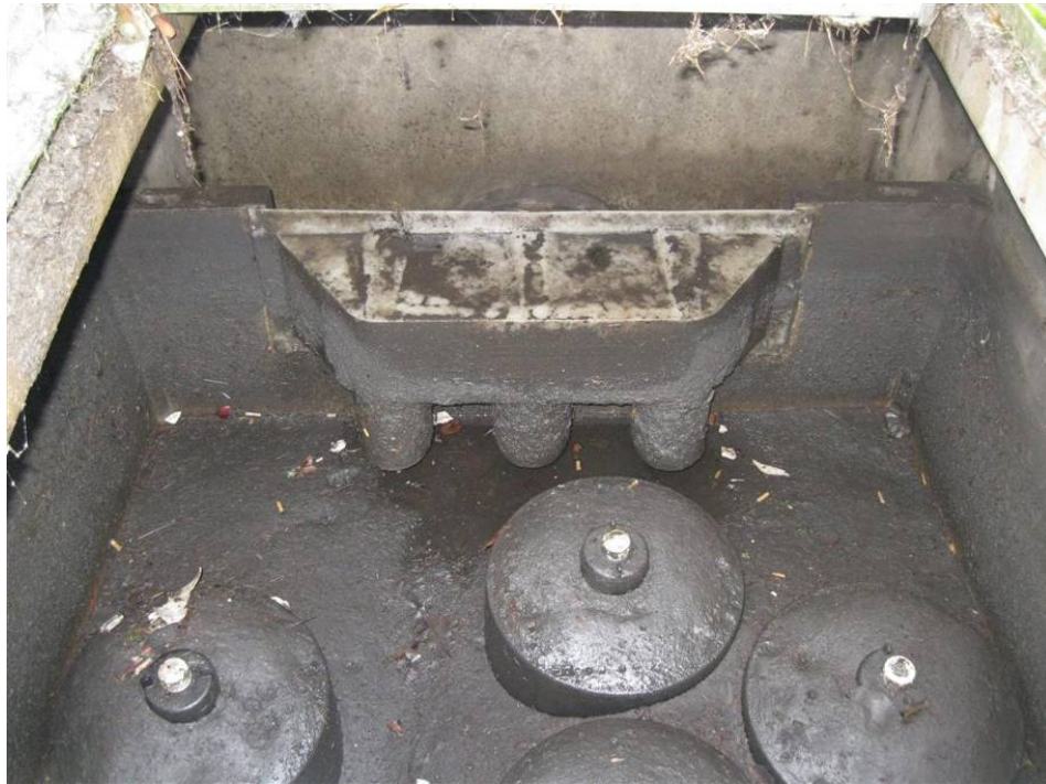
Photo 3: Looking inward at the overflow riser and hood – facility outlet; Vault 2.
