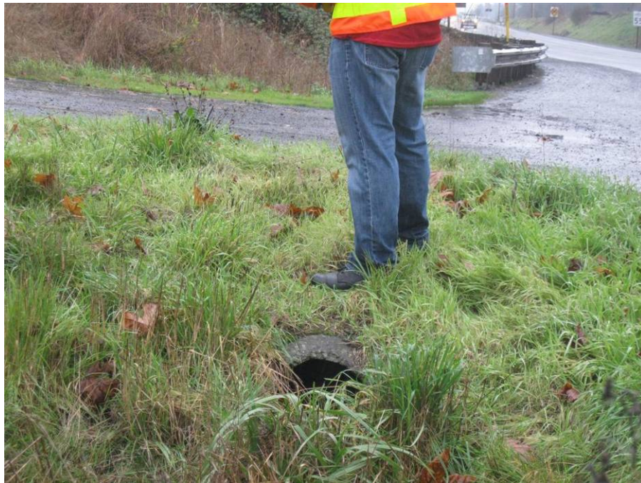
Photo 2: Looking north at the culvert outlet to the swale located north of this point.
