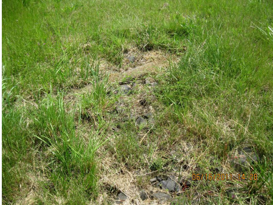
Photo 1: A view of the riprap and small 6" x 3" concrete knee wall flow spreader.
