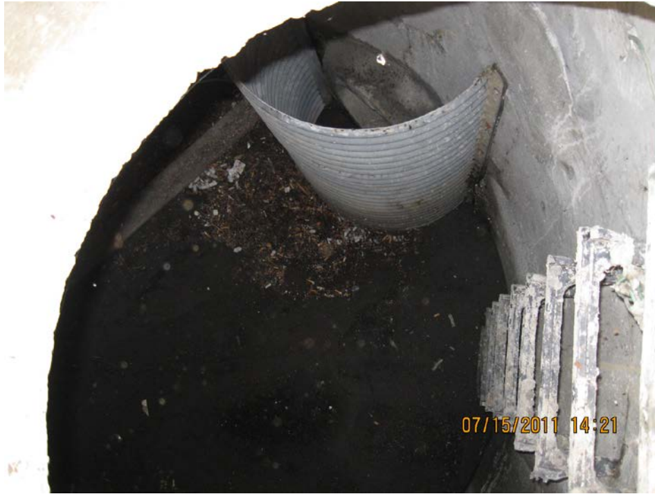
Photo 3: Looking inside of the flow control manhole at the terminus of the detention pipe facility; Point D on Operational Plan; Appendix A.
