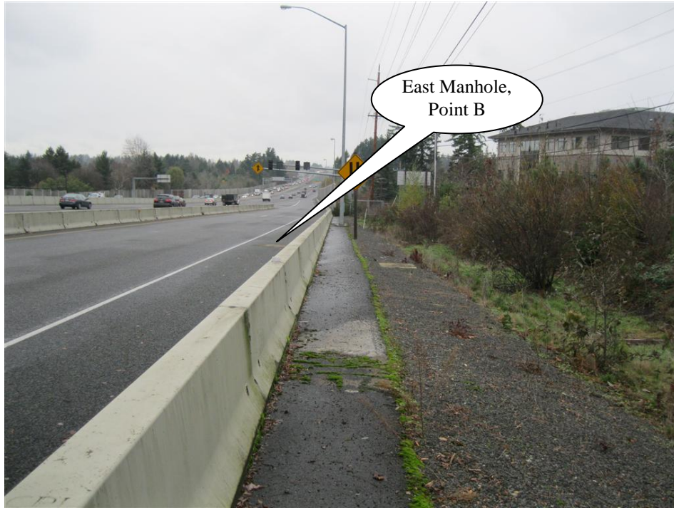
Photo 1: Looking west with US26 (Hwy 047) to the left, and the east manhole of detention facility; Point B on Operational Plan. Water quality facility DFI D00177 is to the right.
