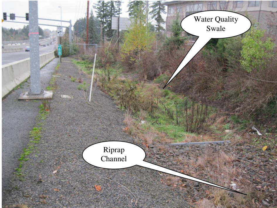
Photo 3: Water quality swale looking west. Riprap channel with flow spreader in foreground.
