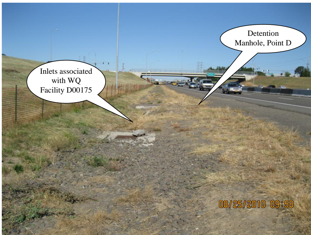
Photo 2: Detention manhole, Point D, and Inlets associated with WQ Facility D00175. Photograph is looking west.
