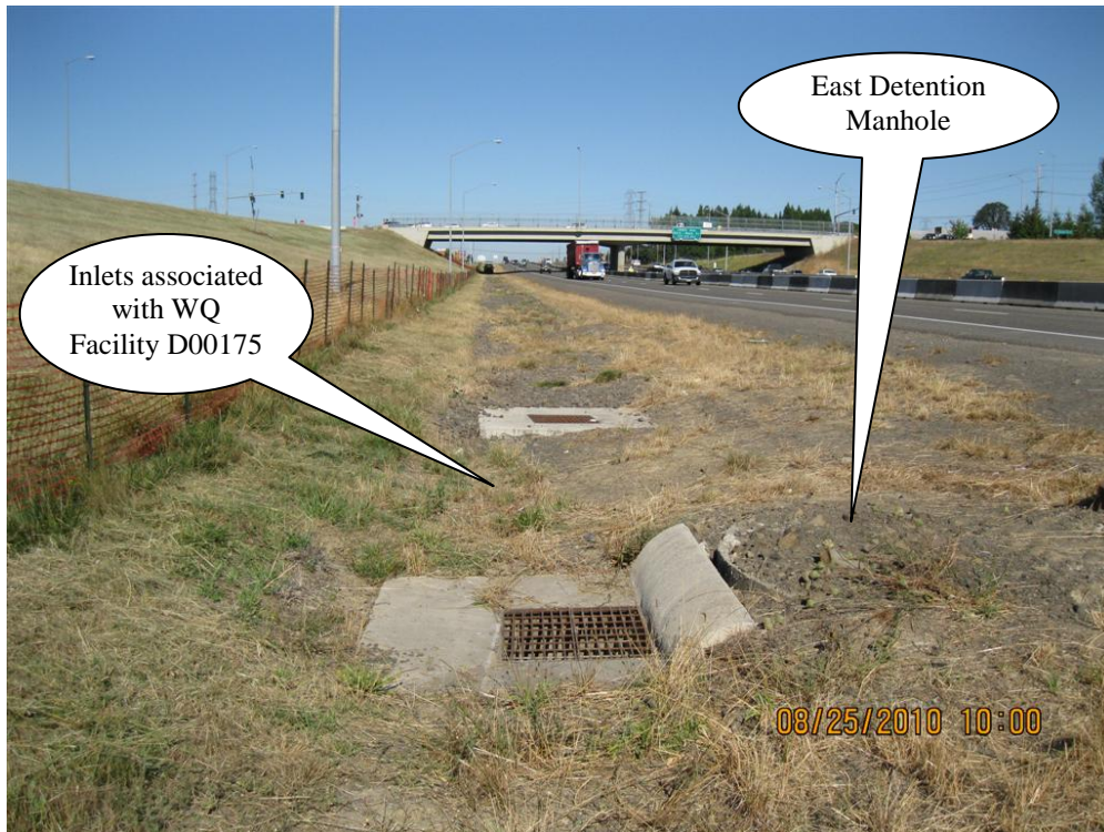
Photo 3: East detention manhole and Inlets associated with WQ Facility D00175. Photograph is looking west.
