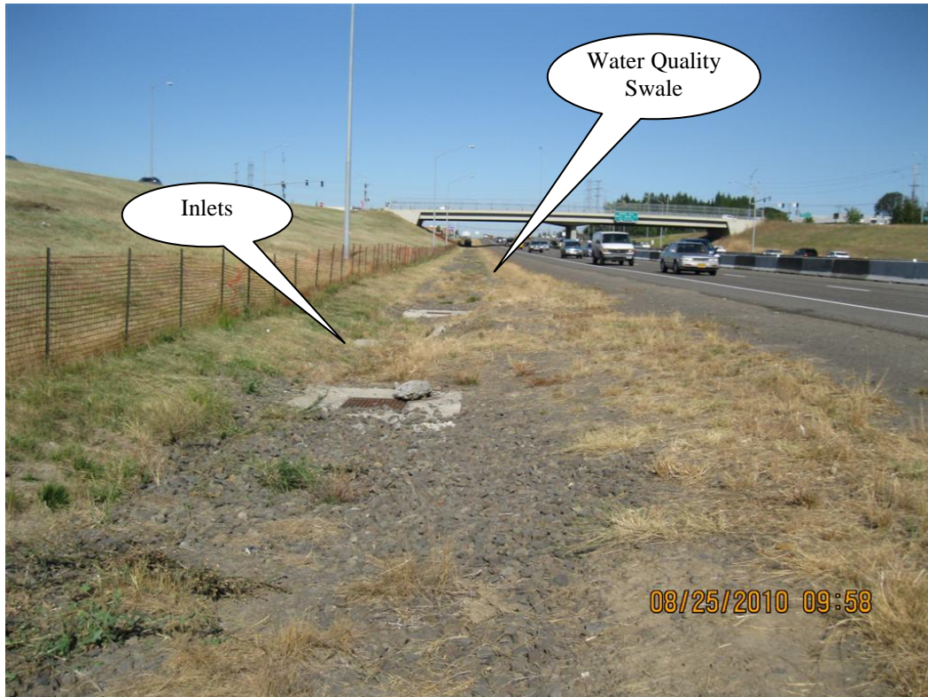
Photo 2: Water quality swale at the midpoint looking west.
