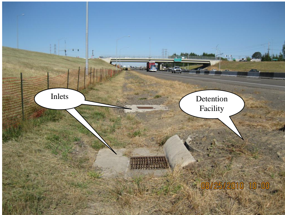
Photo 3: Swale Inlets A and B (Points A and B) looking west. The large manhole adjacent to Inlet B is associated with the detention facility D00176.
