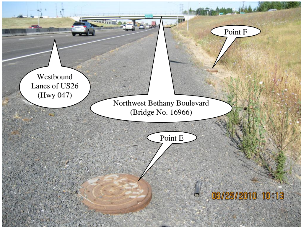
Photo 3: The westernmost manhole for the detention facility contains the flow control device ( Point E ). After detention the water is directed by a 24-inch storm pipe to a manhole ( Point F ). Photo taken facing west.
