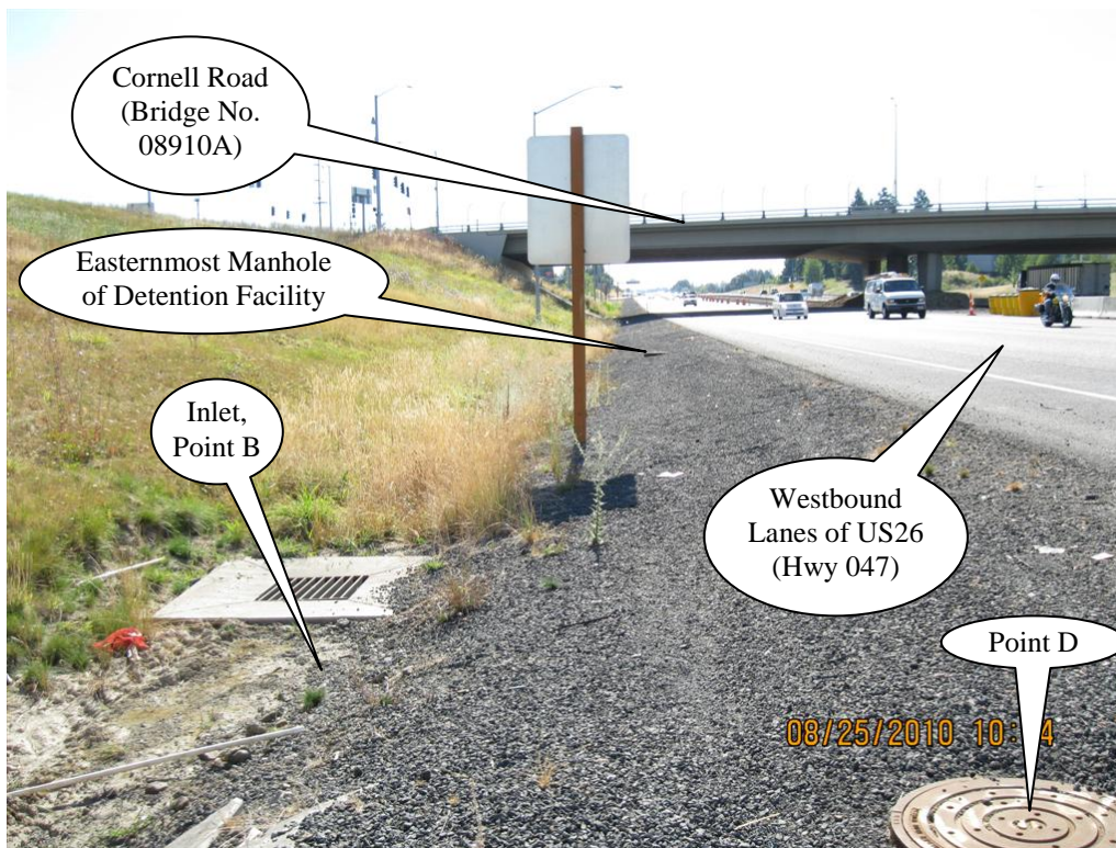
Photo 2: The central manhole of this detention facility is shown in foreground ( Point D ). The easternmost manhole of the detention facility is shown in the background. Westbound lanes of US 26 (Hwy 47) are on the right. Photo taken facing east.
