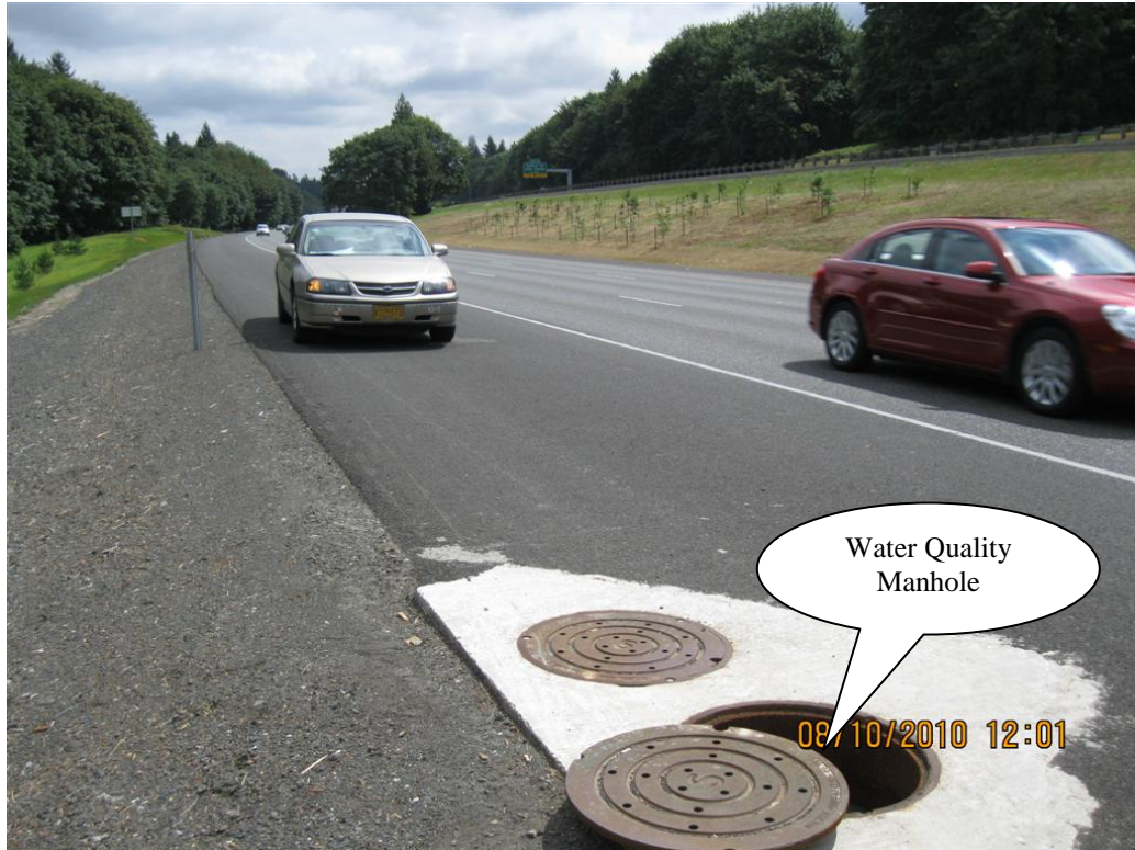
Photo 2: Water quality manhole (D00147), located south of the detention facility.
