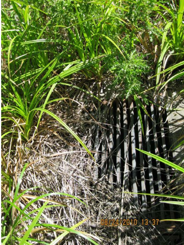
Photo 5: Outlet control structure of water quality swale.
