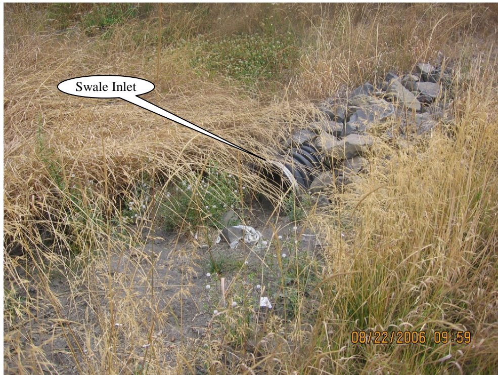
Photo 1: 15-inch storm pipe outfall serving as swale inlet at south end of swale ( Point A ).
