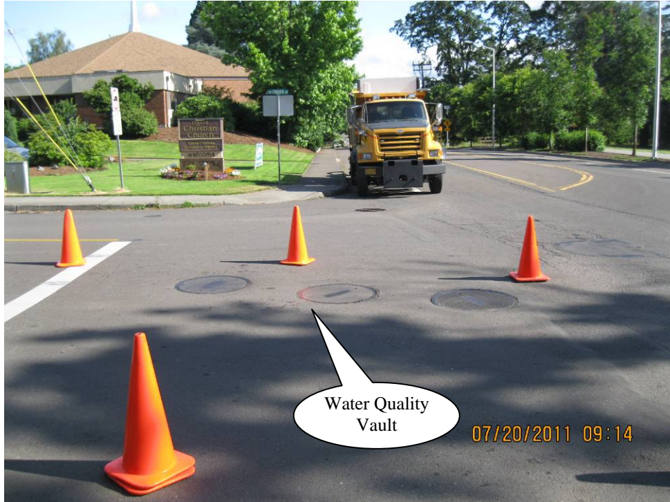
Photo 1: Looking north, this photo depicts the manhole lids of the water quality vault at the intersection of Hall Blvd and SW Omara St.
