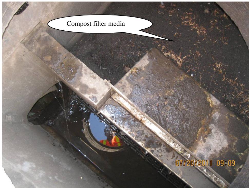
Photo 4: Internal view of water quality vault at the backside of the outlet; Point C Operational Plans.
