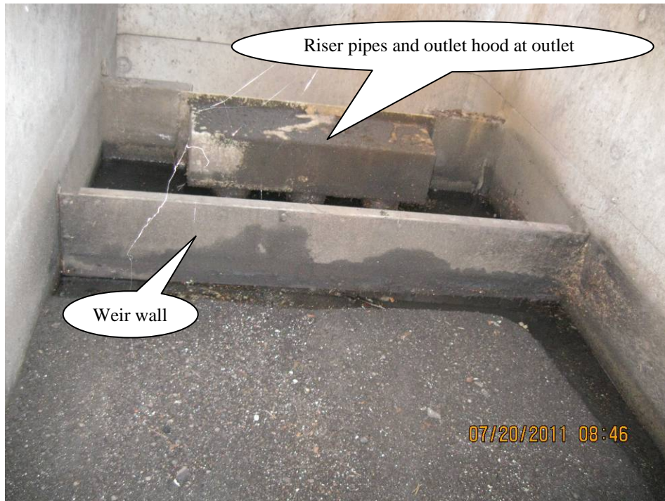
Photo 3: Internal view of water quality vault of the riser pipes and outlet hood near the outlet; Point C Operational Plans.
