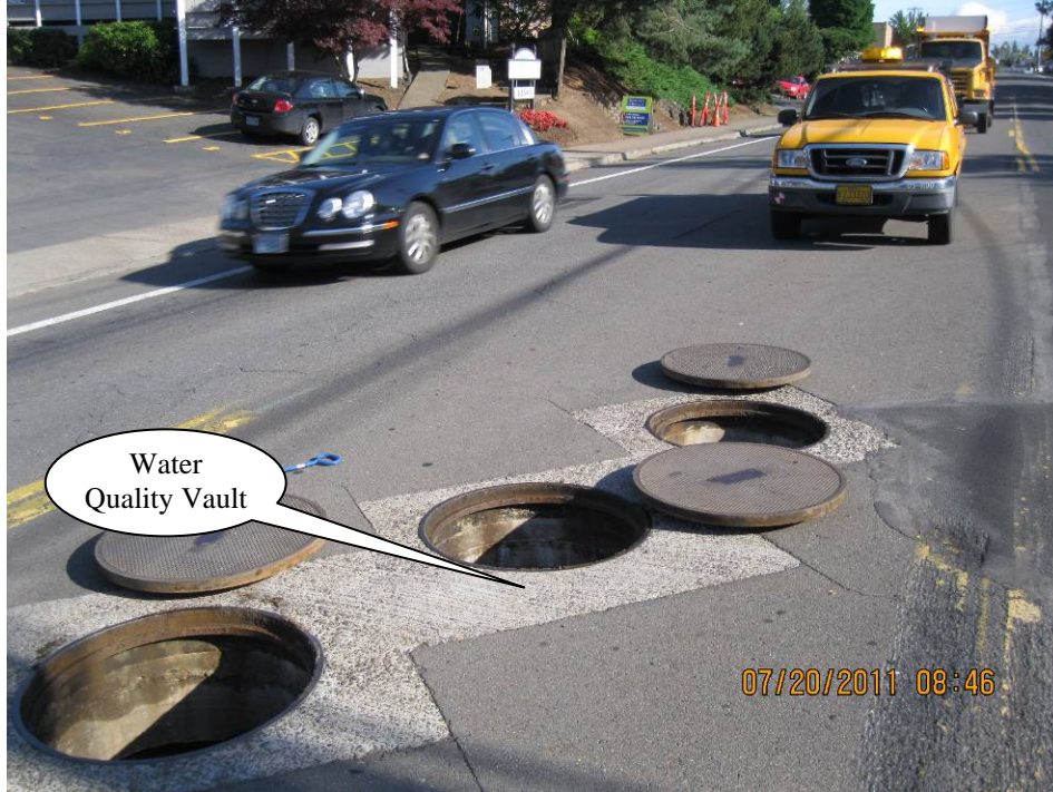
Photo 1: Looking northwest, this photo depicts the open manhole and lids of the water quality vault located within Hall Blvd. at Knoll Drive.
