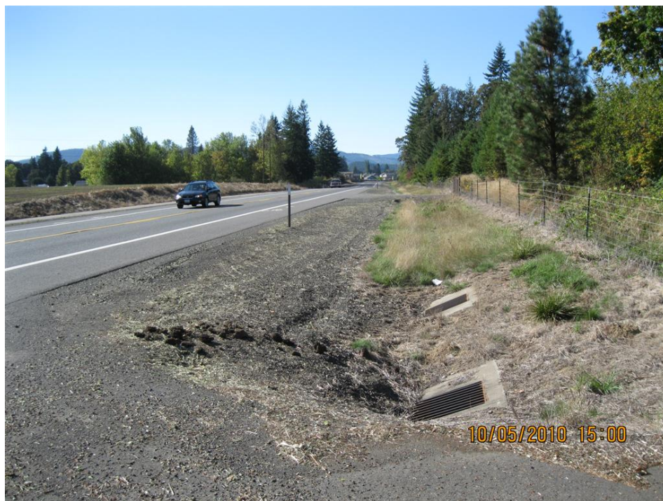
Photo 4: US47 (Hwy 102) located north of the access pullout. Runoff along the north side flows within a roadside ditch as shown. Runoff along the south side is conveyed by a concrete curb.
