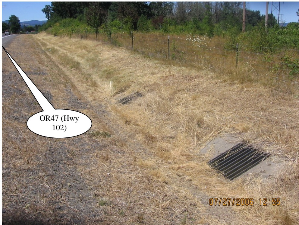
Photo 4: WQ Swale inlets just northwest of access pullout. Photograph is looking to the northwest.
