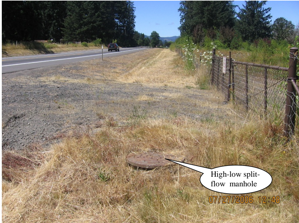
Photo 6: High-low split-flow manhole, looking northwest.
