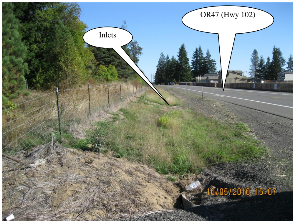
Photo 2: Roadside drainage ditch on north side of OR47 (Hwy 102). Photograph is looking towards the east.
