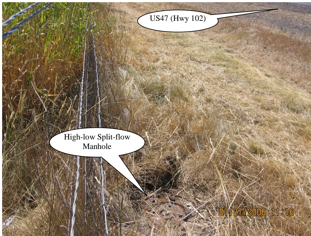
Photo 6: Split flow manhole located immediately adjacent to access control fencing.
